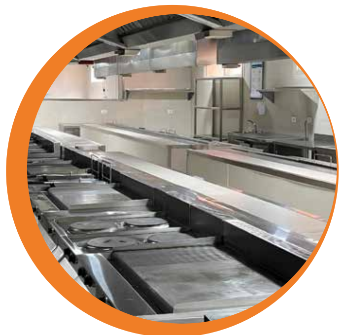
Figure 15: Practice kitchen funded and installed by the private sector partners. Source: Authors
