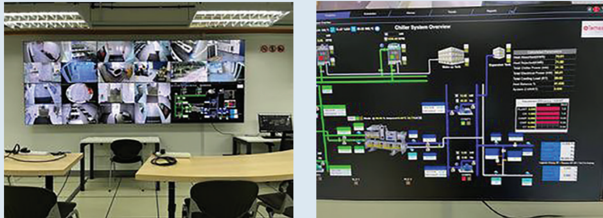
FIGURE 15. TV MONITORS SHOWING THE FUNCTIONS AND NETWORKS OF THE TP BUILDING
