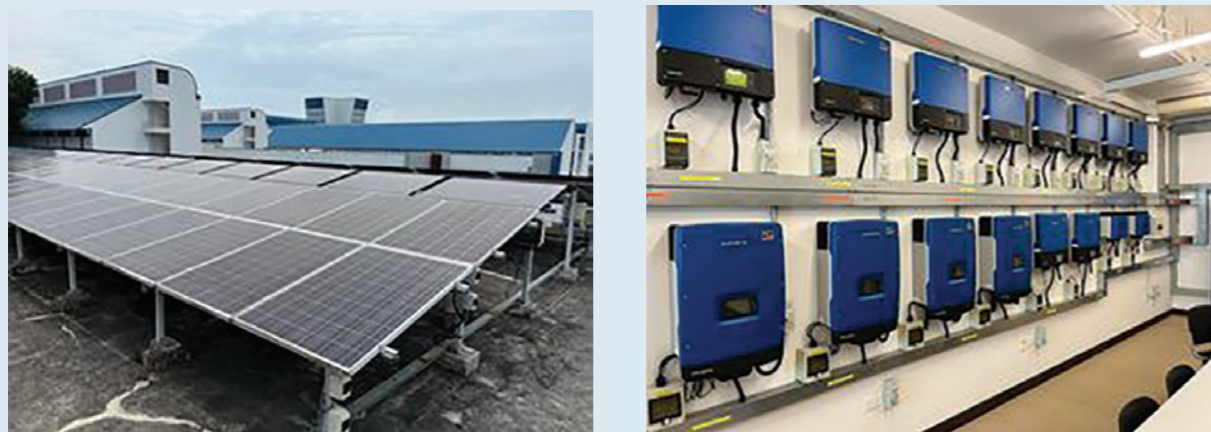
FIGURE 13. SOLAR PANELS (LEFT) AND CONTROL ROOM (RIGHT)
